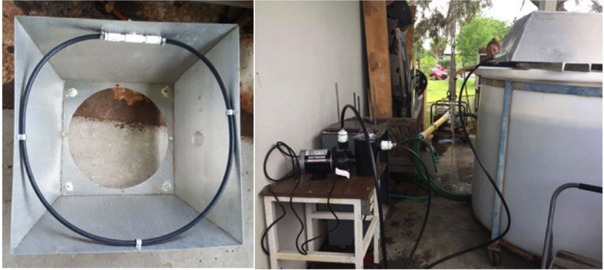
Figure 5: Active Jet Setup with Pool Pump and Irrigation Hose
