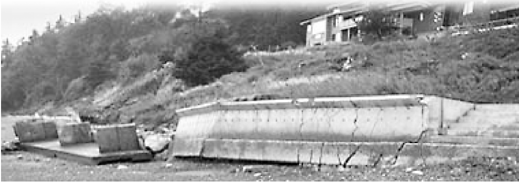
Figure 6. Failed bulkheads and large slide on Whidbey Island (Washington Department of Ecology http://www.ecy.wa.gov/programs/sea/pugetsound/building/bulkhead.html )
