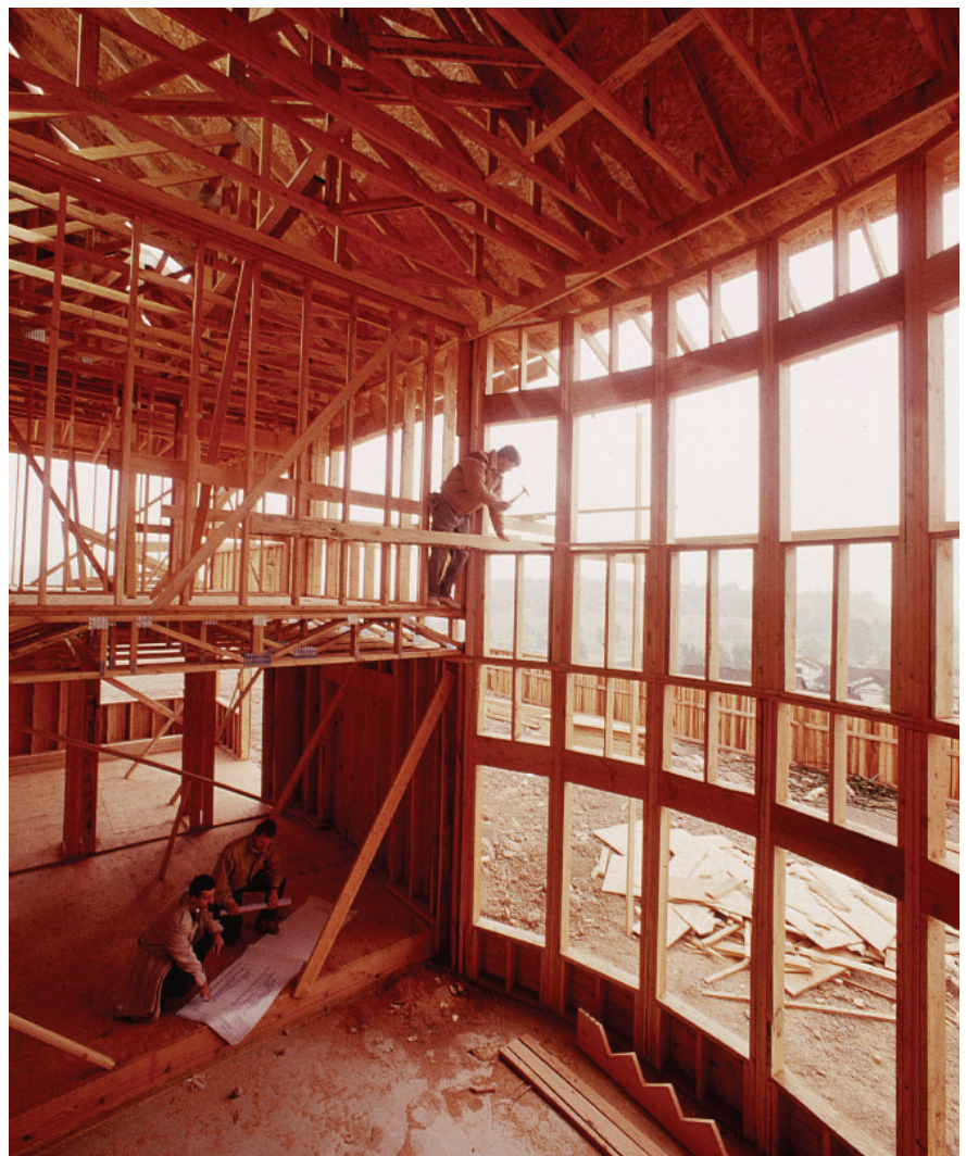
Workers construct an energy efficient house in Rocklin, California, a city just north of Sacramento. California's climate change policies encourage builders to build green.
