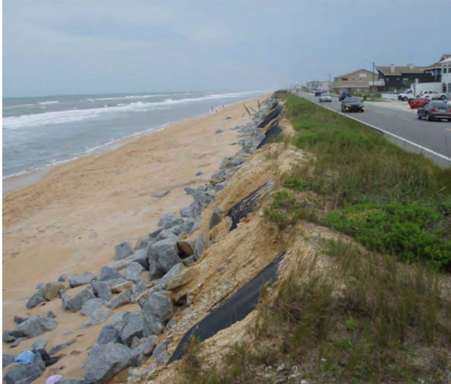
FIGURE 3-1 An eroding beach adjacent to State Road A1A in Flagler County, Florida, recently under study by the USACE for additional hurricane and storm damage risk reduction.
