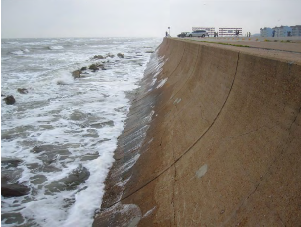
FIGURE 1-6 Seawall along the coast of Galveston Island, Texas. SOURCE: Photo courtesy of Melanie Fitzpatrick, Union of Concerned Scientists.
