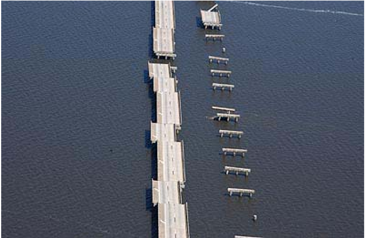
Figure 3: I-10 Bridge over Escambia Bay, Florida after Hurricane Ivan, 2004
