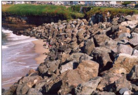
Figure 1. Revetment in Santa Cruz, California (note the absence of a sand beach). 8
