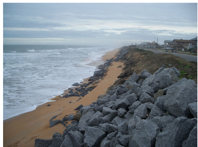
Fig. 2 Failing rock revetment at South 17th Street, Flagler Beach, Florida. Author’s Photo, January 2014
