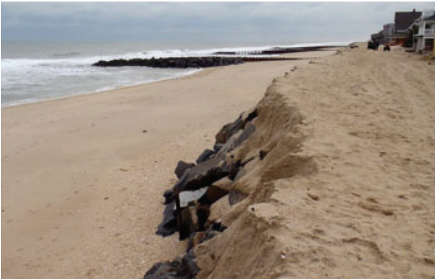
FIGURE 3-4 Relic seawall in Bay Head, New Jersey, that was buried beneath a dune and uncovered during Hurricane Sandy.
