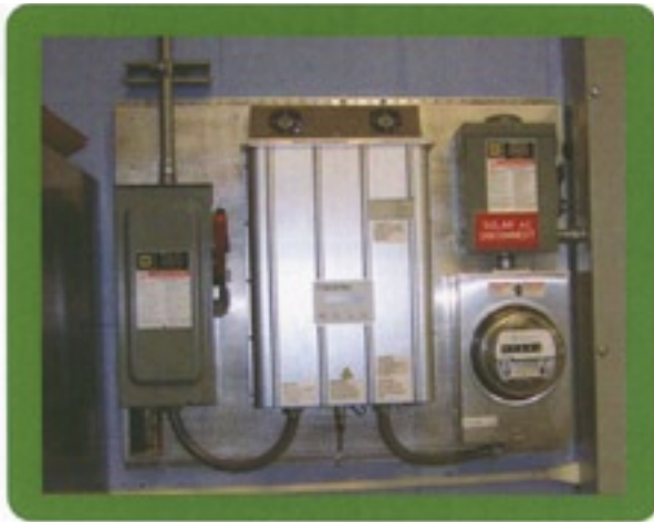
The solar inverter in the Murchpy school science lab
