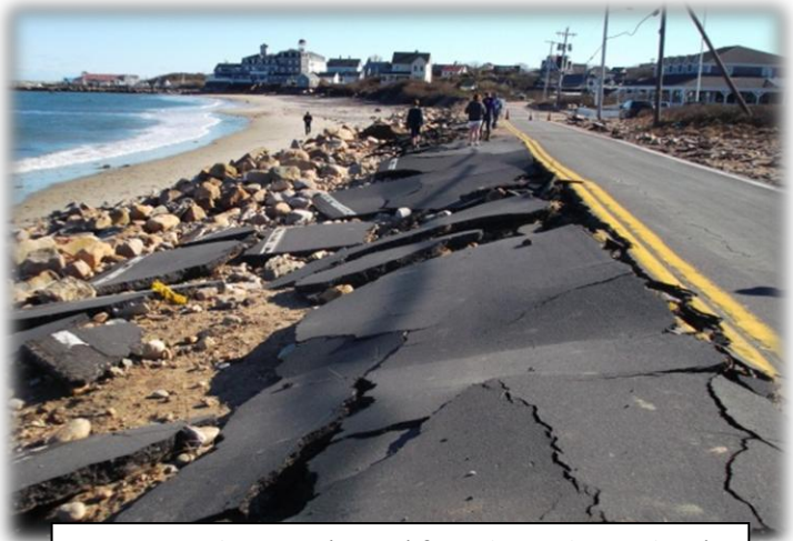
Damage to Corn Neck Road from Super Storm Sandy October 2012
