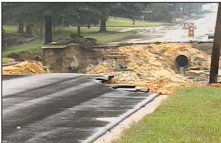
Road washout from heavy rainfall event.
