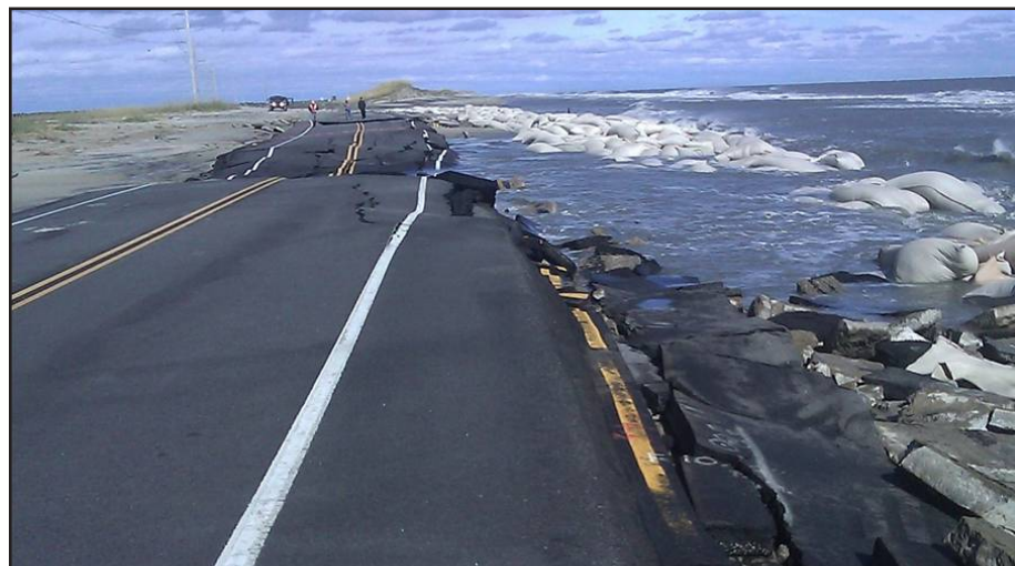
N.C. Highway 12 after Superstorm Sandy wrecked sandbag structures built to protect it. Photo courtesy N.C. Department of Transportation
