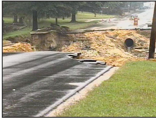
Road washout from heavy rainfall event.
