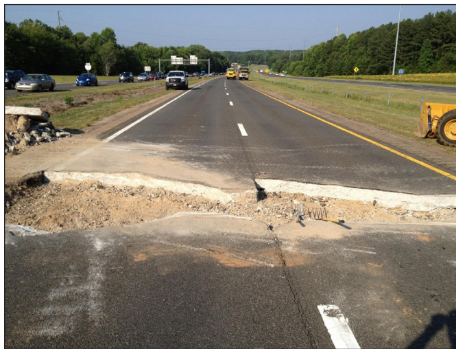
"Pavement buckling" is also known as a blow up or blow out, caused by heat expansion of the concrete slabs. If the joints are not wide enough to accommodate the expansion, the concrete "tents up." It is relatively rare.
