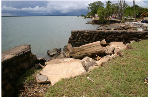
Fig. 6 Damage to the sea wall caused by a stormtides on Saibai in 2006 (photo credit: Donna Green)
