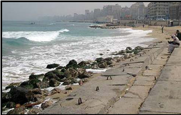
Figure 4: Weakness of the erected sea wall on Alexandria shore.
