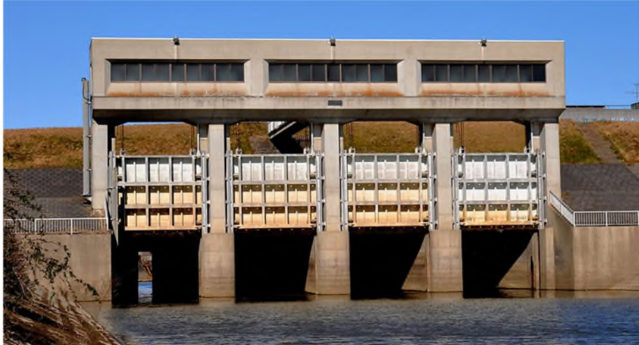
Figure 5-14: Example weir gate system (Pxfuel 2020)
