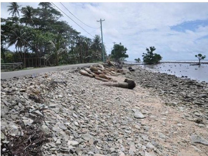
Gradual coastal erosion threatens housing along the coastline in Malem, July 2012 (Source: Doug Ramsey)
