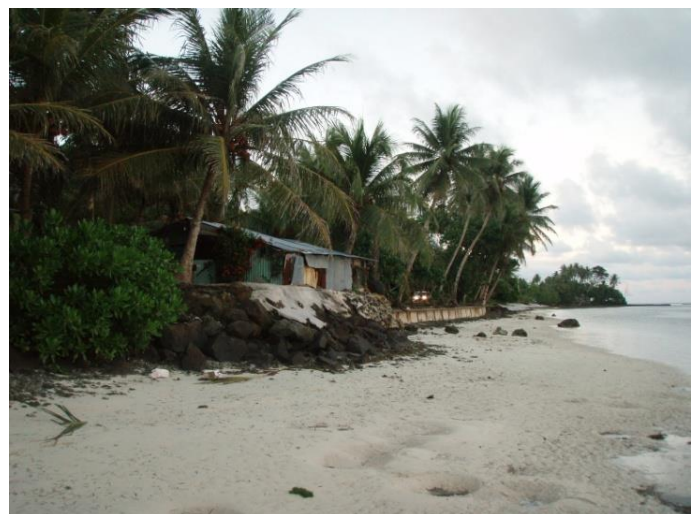
Seawall covered with cement to protect a house in Lelu, Kosrae. Photo: Iris Monnereau
