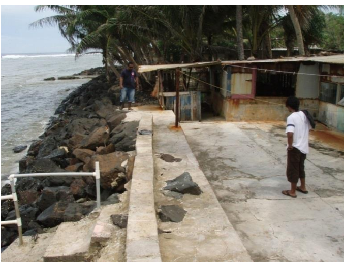
The seawall behind the house and bakery of Kilafwasru Kilafwasru and Sepe Kilafwasru in Malem (box 4.5). Photo: Iris Monnereau
