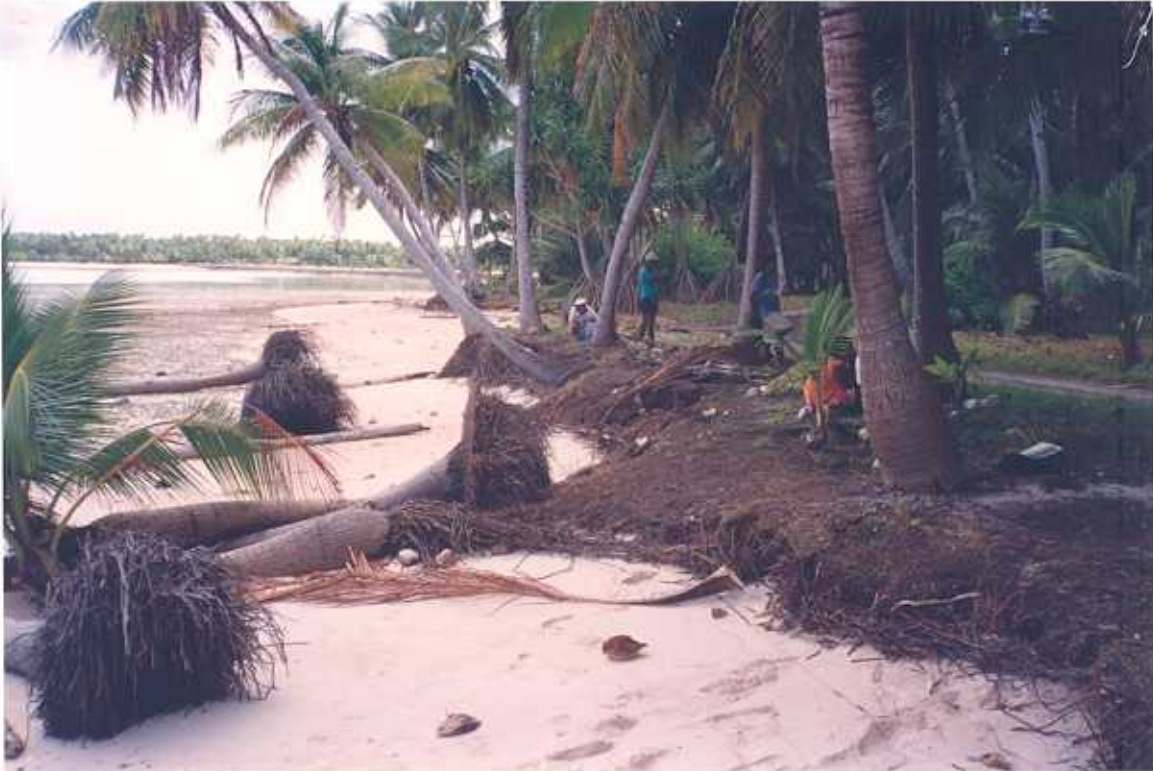
Figure 8. Nikutiri Island, Tabiteuea South. View north along lagoon shoreline at beach profile site showing erosion as indicated by beach scarp and fallen coconut trees. Erosion is also undermining the road. Causeway shown in Figure 9 is visible in the distance.
