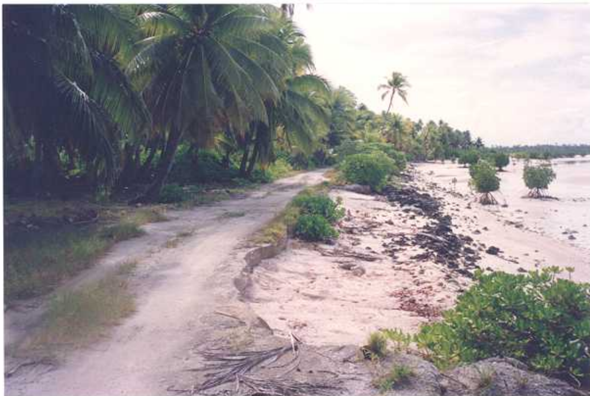
Figure 34. Rotima Island (Site 1: airfield road), Nonouti. View southeast showing erosion of airfield road approximately 30 m south of terminal under construction on date of survey.
