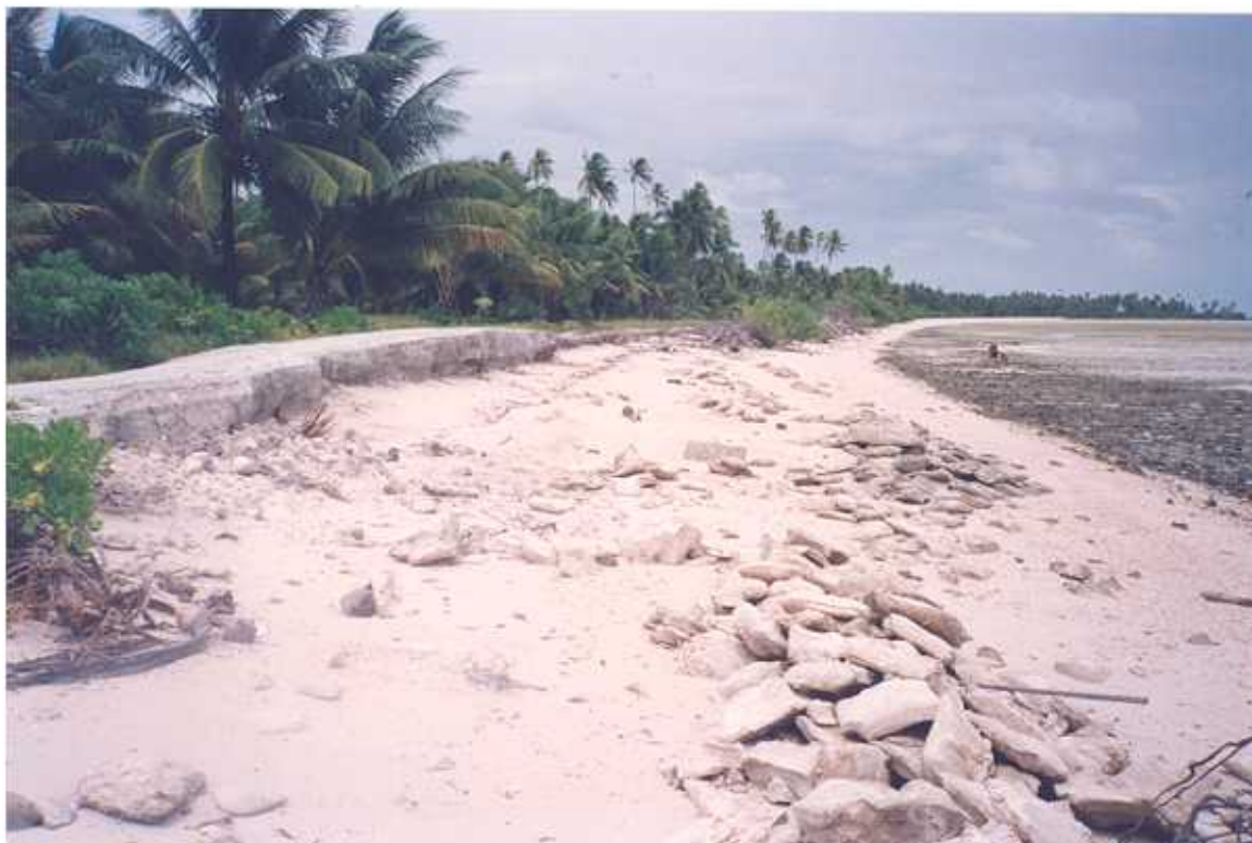
Figure 37. Buariki Village, Nonouti. View southeast along lagoon shoreline. Erosion indicated by beach scarp undermining road and remains of seawall constructed from concrete filled sandbags. Reef is covered by thin veneer of sand.
