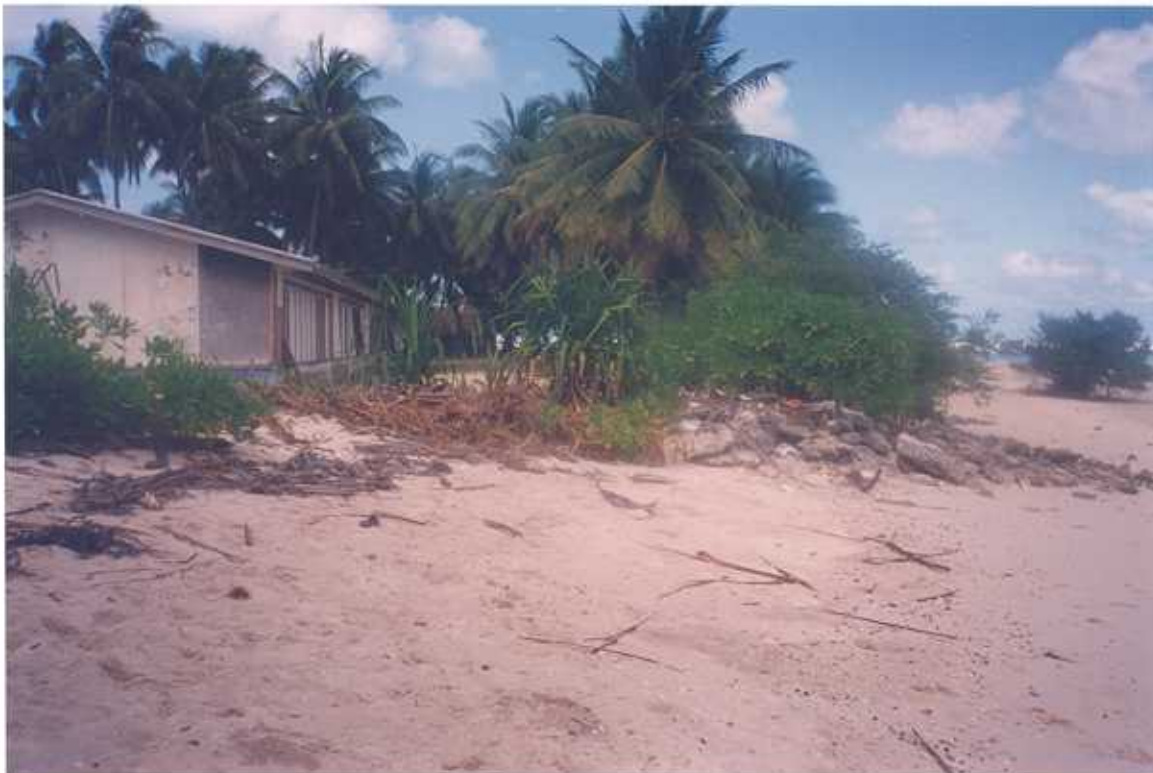
Figure 17. School at Tewai, Tabiteuea South. View southwest along inter-island channel shoreline showing condition of eastern end of seawall and proximity of school building to the shoreline.
