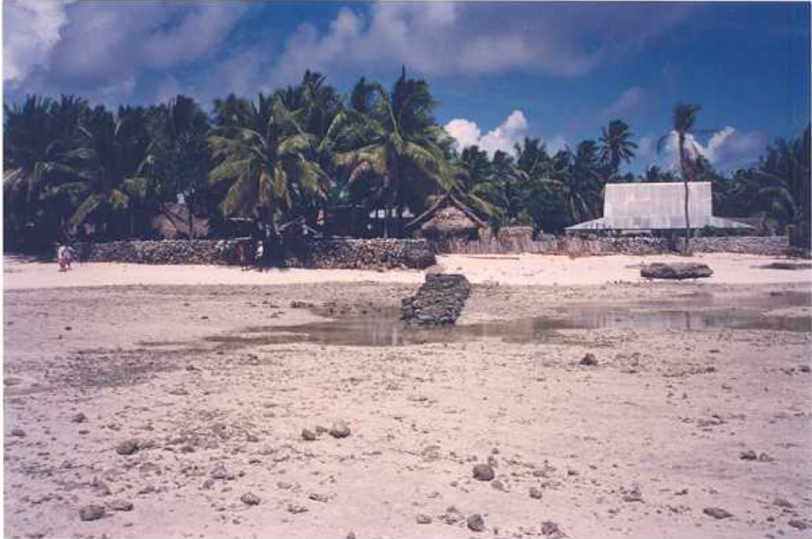
Figure 21. Onotoa, Tabuarorae Village. View southeast from reef flat showing east gabion basket groyne and extensive seawall construction. Photo taken approximately 40 m west of Figure 20.
