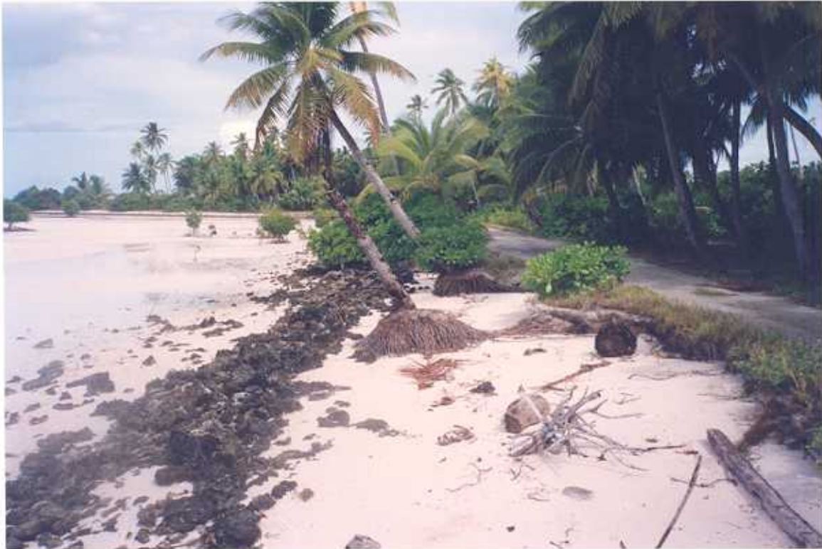
Figure 33. Rotima Island (Site 1: airfield road), Nonouti. View northwest along lagoon shoreline. Coastal erosion indicated by exposed roots of coconut trees, encroachment of beach on road and remains of seawall constructed at original position of shoreline.
