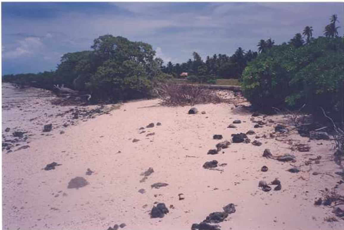
Figure 36. Rotima Island (Site 2: west end of airfield), Nonouti. View northwest at east end of gabion basket seawall shown in Figure 35. Erosion of shoreline is undermining existing road.
