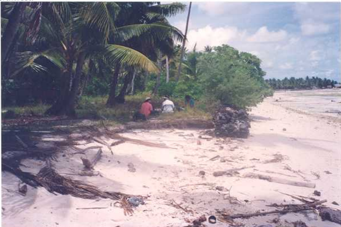
Figure 41. Tanimainiku (Beach Profile: 1), Abemama. View southeast along lagoon shoreline at location of beach profile. Note erosion of shoreline behind existing seawall position (right of photo centre).
