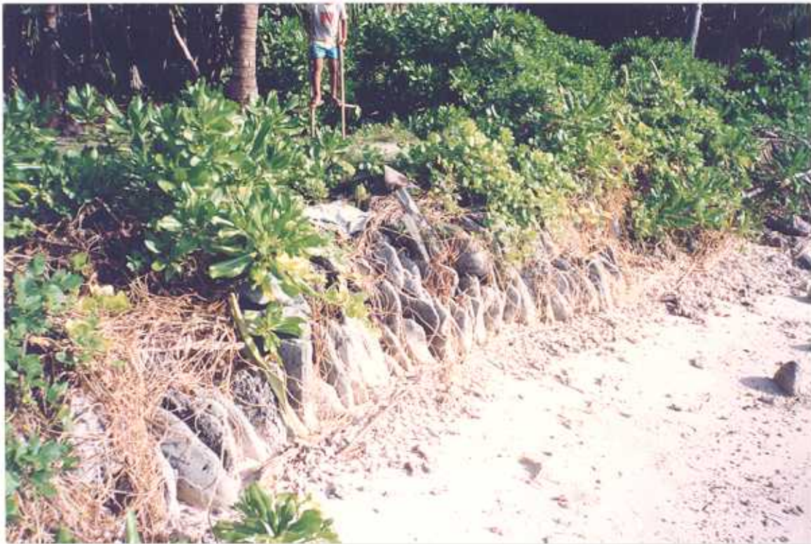
Figure 27. Tetabakea (Site 2), Temotu Island, Nonouti. Beach below road showing traditional seawall constructed of disc-shaped coral boulders. The boulders are stacked vertically. This type of seawall is only suitable for sites of low wave exposure.
