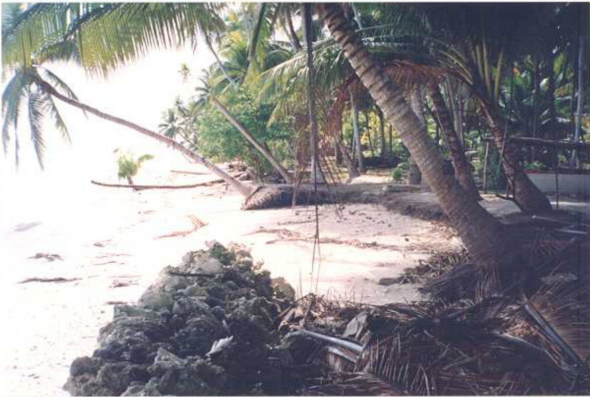
Figure 3. Eita District, Tabiteuea North. View north of beach profile location Eita-1. Note coastal erosion as indicated by beach scarp, fallen coconut trees and remains of coral boulder seawall in the foreground. Seawall foreshore protection makes up less than 5 % of the shoreline in this area.
