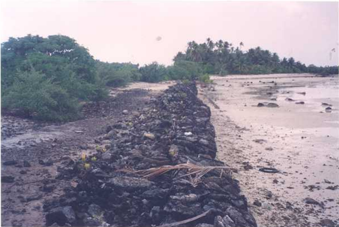
Figure 35. Rotima Island (Site 2: west end of airfield), Nonouti. View southeast along gabion basket seawall constructed to protect land reclaimed for airfield. According to local island sources the seawall was built in 1990.
