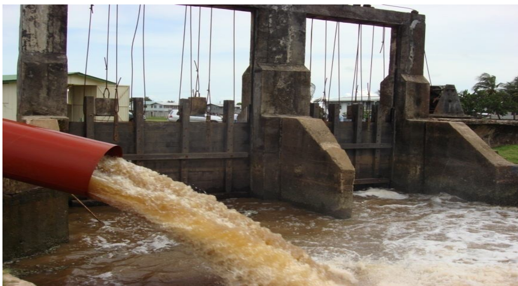
Figure 43: Guyana: Pump and sluice
