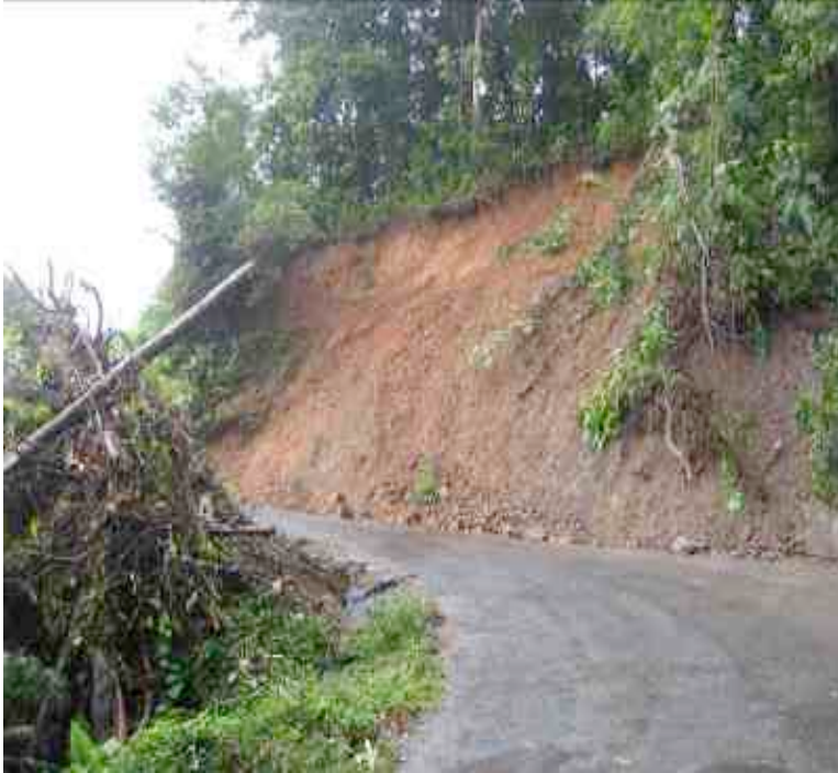
Figure 12: Landslide in Pont Casse area
