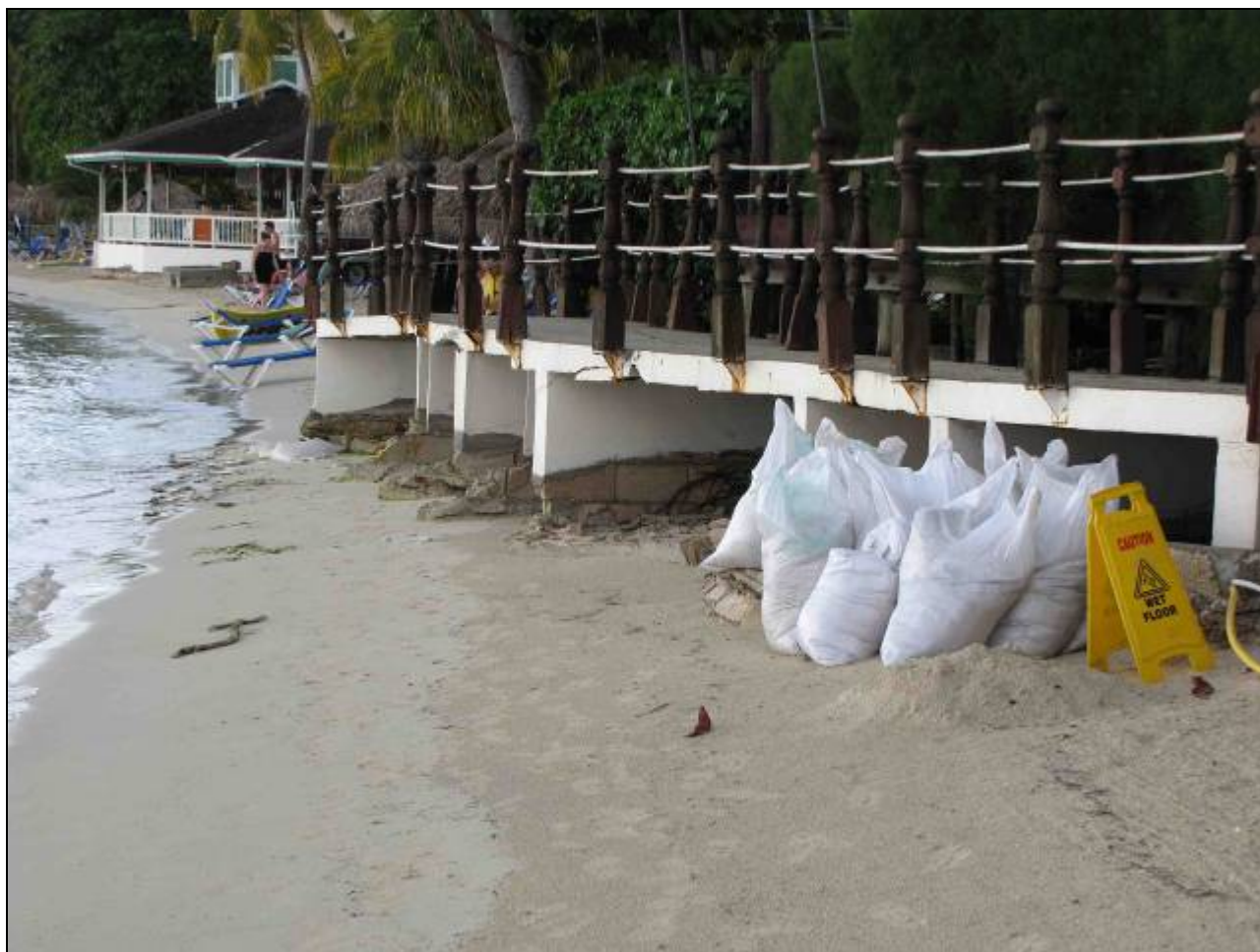
Figure 3.7-3: Erosion Damage to Tourism Infrastructure in Long Bay
