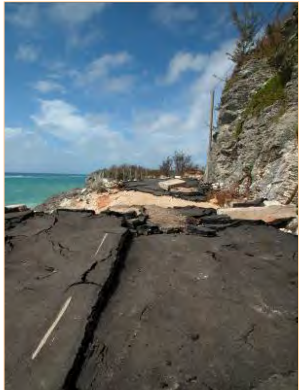
Photograph 4. Showing structural damage to South Shore Road caused by Hurricane Fabian.
