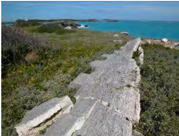
Photograph 5 showing the collapsed wall of Southampton Island Fort after Hurricane Fabian in 2003.
