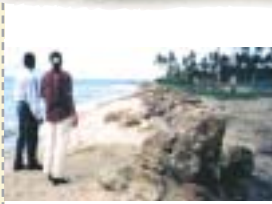
Planning officials inspecting a newly constructed rock revetment at Pinney's Cotton Ground, 1999
