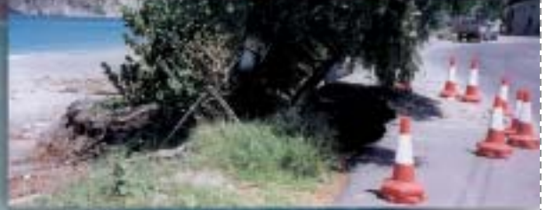
Road damage at Carr's Bay after Hurricane Georges, 1998
