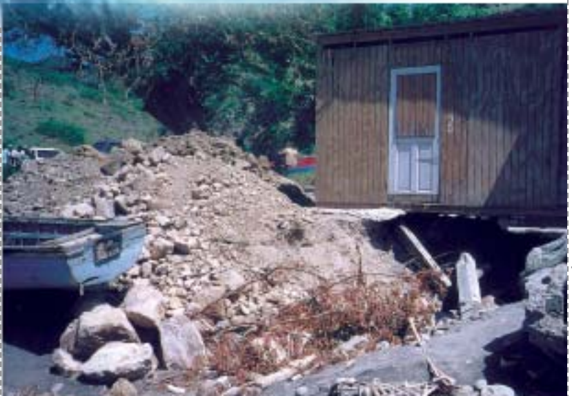
The foundations of this house at Carr's Bay were washed out during Hurricane Georges, 1998
