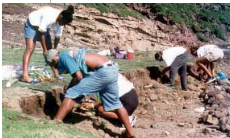
Students building stone barriers and planting cacti to prevent soil erosion, Park Bay, Bequia, St Vincent and the Grenadines 1997.
