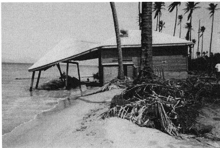
This restaurant is a victim of coastline retreat. Construction setbacks should take adequate account of such potential encroachment of the sea.
