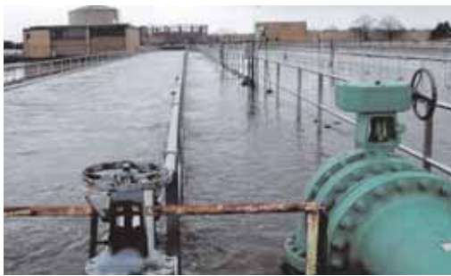
Figure 59: Treatment tanks overflowing at a Bronx Water Pollution Control Plant during March 2001 storm. Unusually high tidal elevations blocked discharge of treated sewage into the East River and caused back-up. (Source: New York City Department of Environmental Protection).
