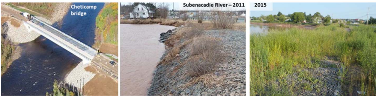
SCOUR PROTECTION AT CHETICAMP BRIDGE PIERS USING ROCK (LEFT), AND ALONG TIDAL SHUBENACADIE RIVER, NS (MIDDLE AND RIGHT) USING ROCK-FILLED GABION MATS. (IMAGE SOURCES: CBCL LIMITED)
