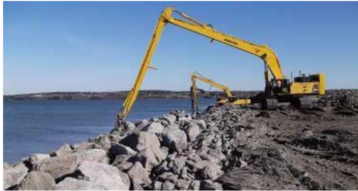
CONSTRUCTION OF A REVETMENT AT SYDNEY HARBOUR, NSW, CONFINED DISPOSAL FACILITY. (IMAGE SOURCE: VINCENT LEYS, CBCL LIMITED)
