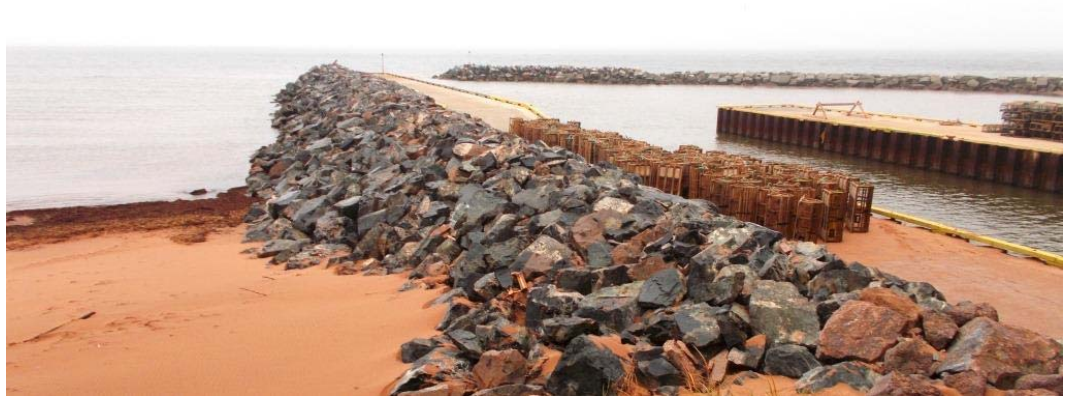
BREAKWATERS AT SKINNERS POND, PRINCE EDWARD ISLAND. (IMAGE SOURCE: VINCENT LEYS, CBCL LIMITED)
