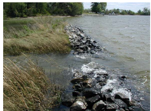
EXAMPLES OF LIVING SHORELINES WITH STRATEGIC ROCK STABILIZATION. (IMAGE SOURCE: DUHRING, BARNARD & HARDAWAY 5 )
