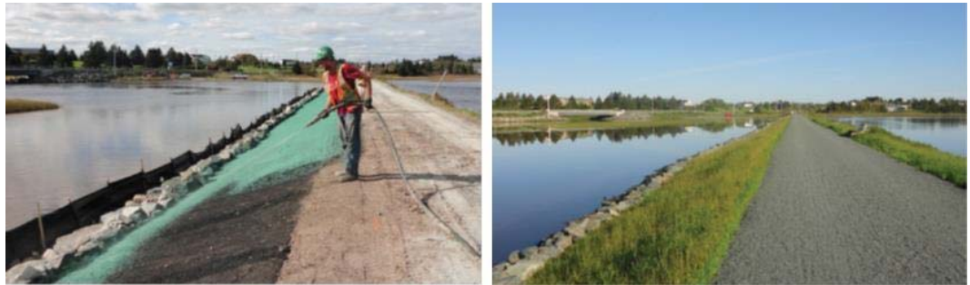
INSTALLATION OF A TURF REINFORCED MAT WITH ROCK TOE UP TO ELEVATION OF HW ALONG COASTAL TRAIL NEAR LAWRENCETOWN BEACH, NS. IT WAS INFILLED WITH HYDRAULICALLY APPLIED MULCH (LEFT), WHICH WAS SELECTED BASED ON THE SITE CONDITIONS. (IMAGE SOURCE: ESANS 1 )
