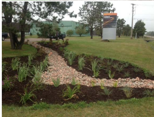
BIO-INFILTRATION ZONE INSTALLATION AT DEBERT INDUSTRIAL PARK, DEBERT, NS (IMAGE SOURCE: TRACEY MACKENZIE)
