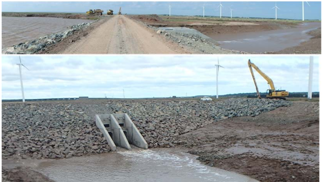
LA PLANCHE RIVER ABOITEAU NEAR COMPLETION, AUGUST, 2015. (IMAGE SOURCE: SUVIR PURSNANI, CBCL LIMITED)
