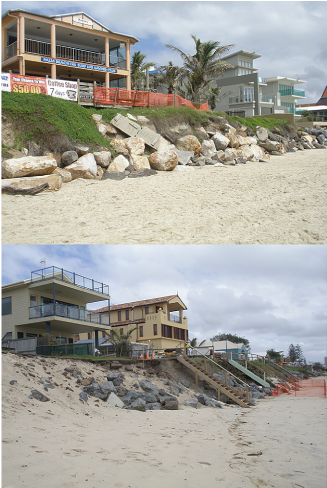
Fig. 10. A-line defences exposed by erosion of covering dune sand and adjacent beach during a storm in May 2009. Photo taken in March 2010.
