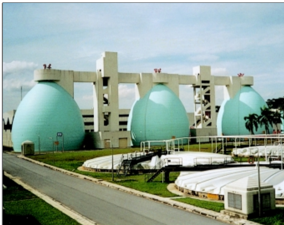
A sewage treatment works where biogas is recovered to produce electricity.
