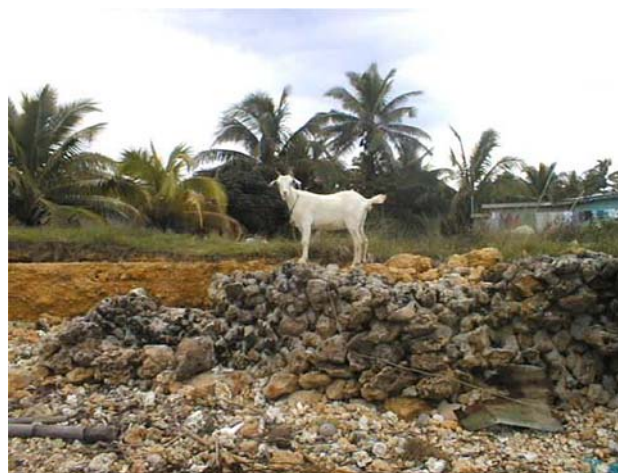
Fig. 9 Part of the degraded seawall protecting the village of Yadua—storm waves penetrate into the land behind the damaged sea wall and erode the coastal flat on which the village lies (Photo: Patrick Nunn, Fiji)
