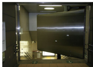
Water stop door
