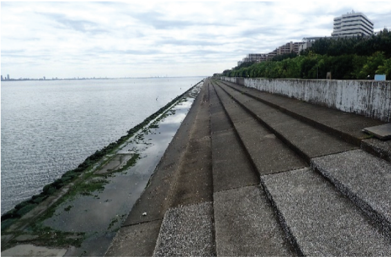
Figure 2. Example of a revetment and seawall on the Urayasu coast in Chiba Prefecture, located at a in Figure 5 .
