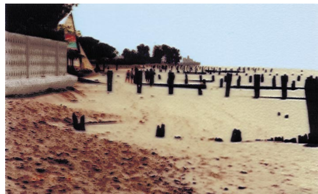
Fig. 4. Damaged groin system that has protected the City of Banjul for more than 40 yr
