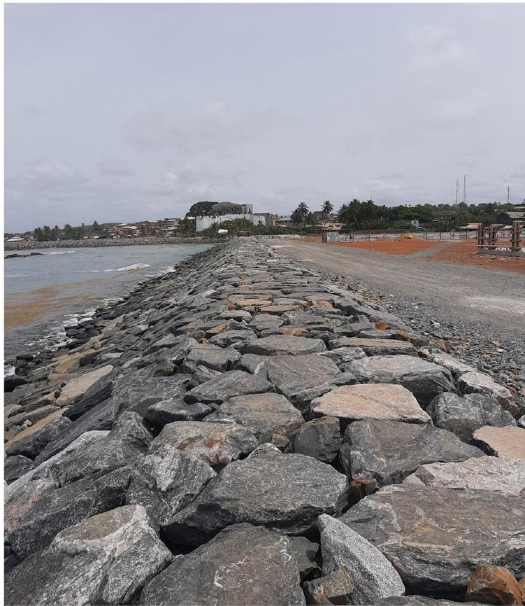
Fig. 10 Construction of the 5 km Axim Sea Defence Project is almost entirely completed
