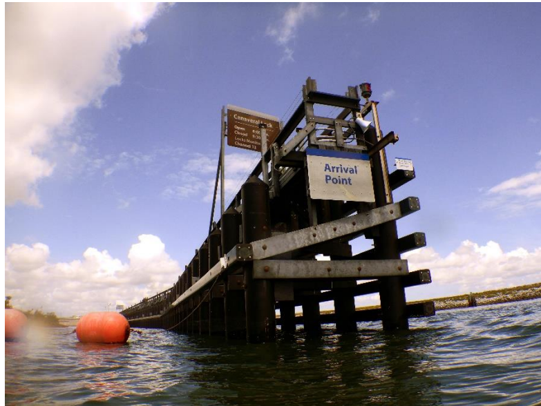
Photograph 5. Canaveral Lock Arrival Point at the western end of the survey area.
